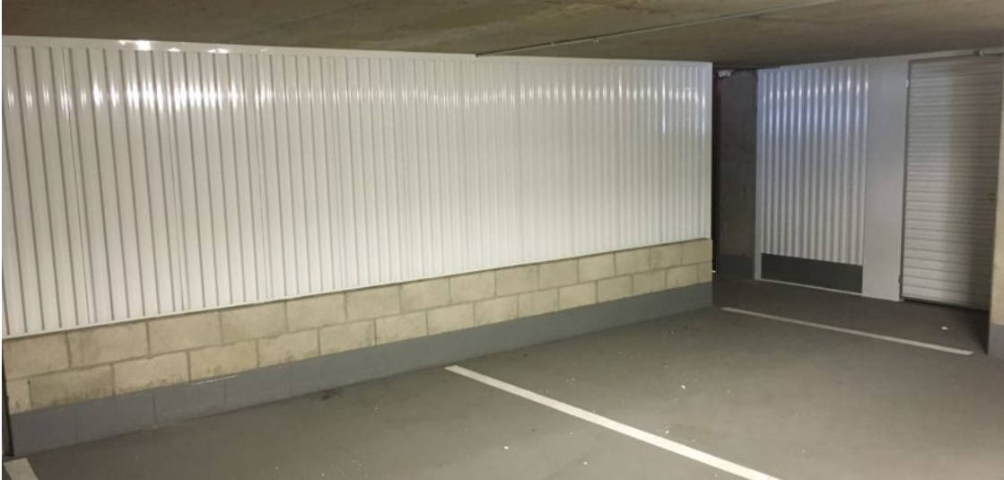
Sample Image – Storage Wall:
