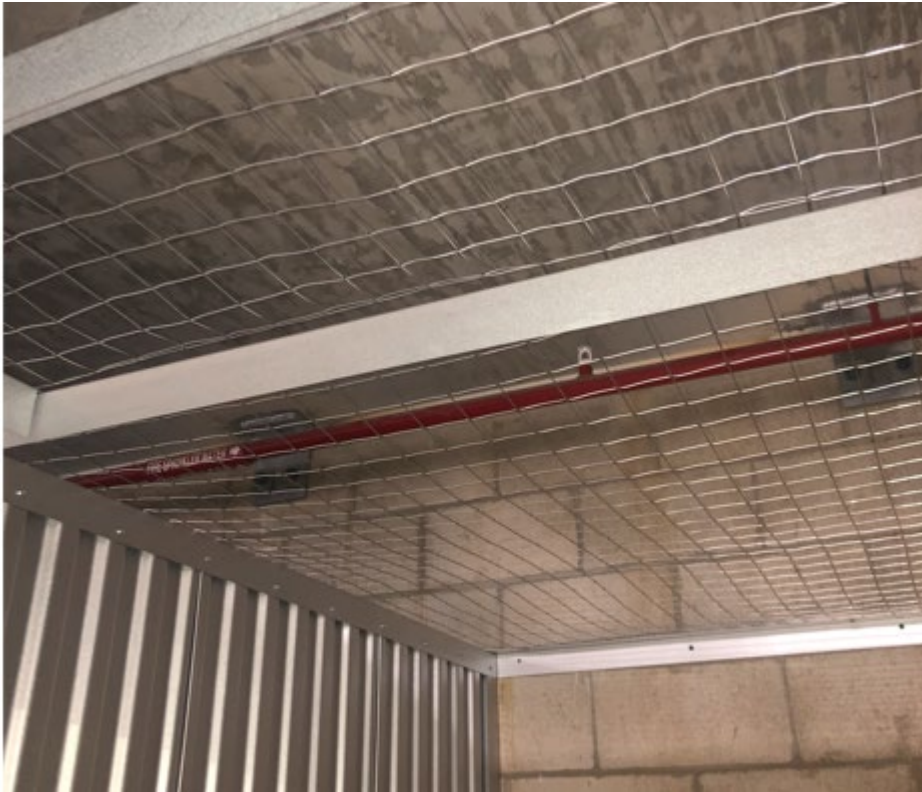
Sample Image – Wire Security Ceiling:
